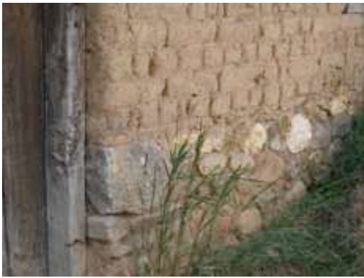
Fig. 4 - The stone foundations that support this mud-brick wall protrude from the ground for protection against humidity Photo: Athanassios Balasas, Nafsika Exintaveloni, 2009
