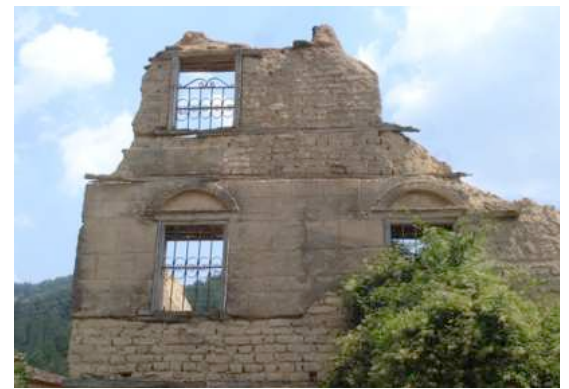
Fig. 9 -The plastering on the walls of this mansion in Antartiko village imitates ashlar stonework, which is a structural element of neoclassical architecture. Photo: Athanassios Balasas, Nafsika Exintaveloni, 2008
